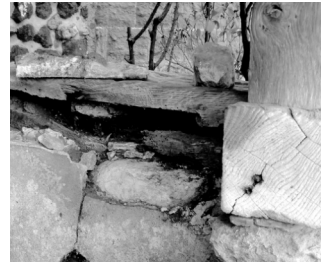
Next step: Strengthen decayed wood, right side of porch.
