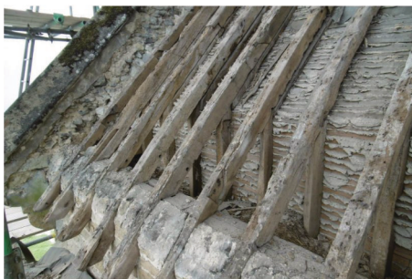
Timbers on the south side of the Chancel roof Images reveal that timbers have been “recycled” from another part of the church or another.
